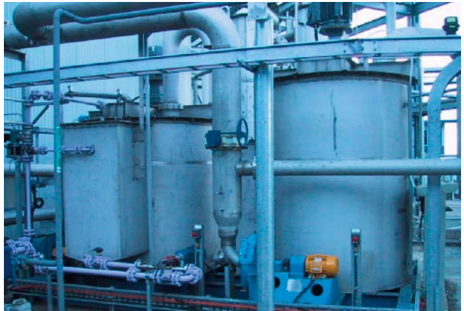
Commissioned in 2005, the GRD Minproc BioGas Purification System handles H 2 S levels ranging from 4000 - 5000 ppmv.
