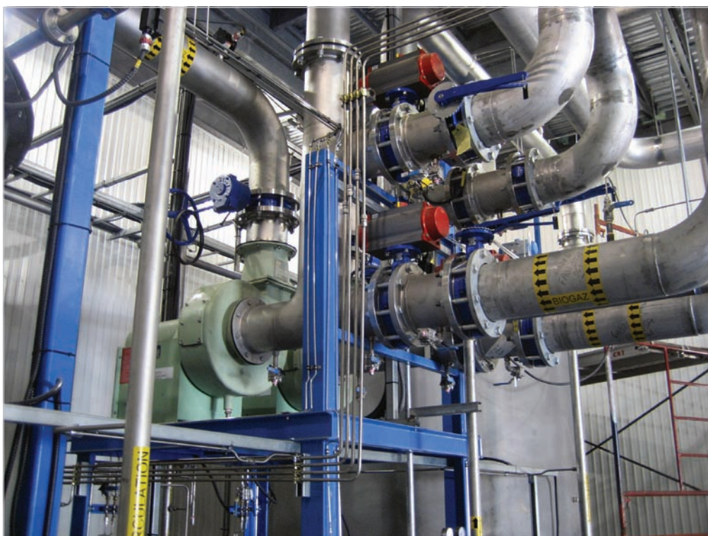
Figure 2. An RGMRM installation
