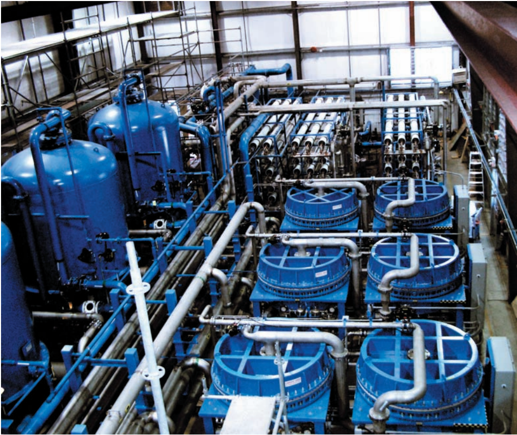
POWERFUL SOLUTION: Eco-Tec's water treatment installation for Ontario Power Generation's reactors in Pickering, Ontario. (Photo: Eco-Tec)
