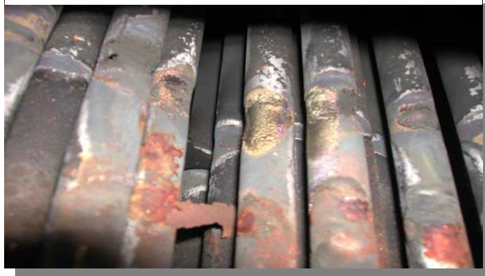
Reboiler piping corrosion caused by HSS build up
