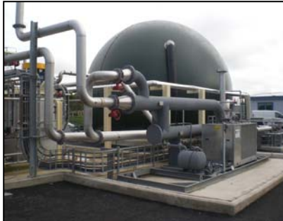
Global Renewables' Thornton Waste Recovery Park integrating Eco-Tec's BgPur biogas purification system.
