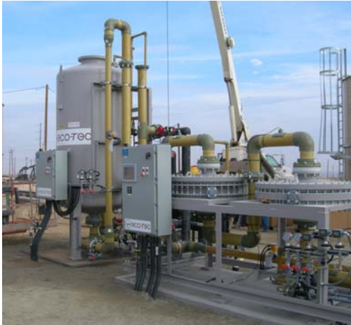
The Eco-Tec RecoPur ® Produced Water Treatment System installed at Seneca Resources includes a Spectrum Filter ™ for oil and solids removal (background) and a Recoflo ® SACPlus softener (foreground).
