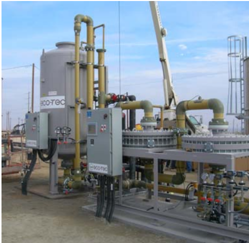
The Eco-Tec system treating produced water at Seneca's North Lost Hills, California operations. Seneca has order two similar systems for its Maricopa operations.
