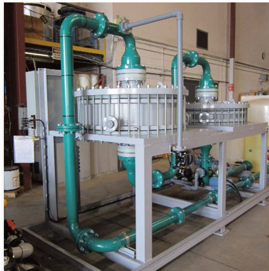
SAC/WAC Skid-mounted Softener
