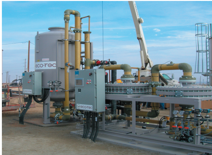
Produced Water Treatment System for Seneca Resources, featuring Spectrum Micro Media Filter in advance of ion-exchange softeners.
