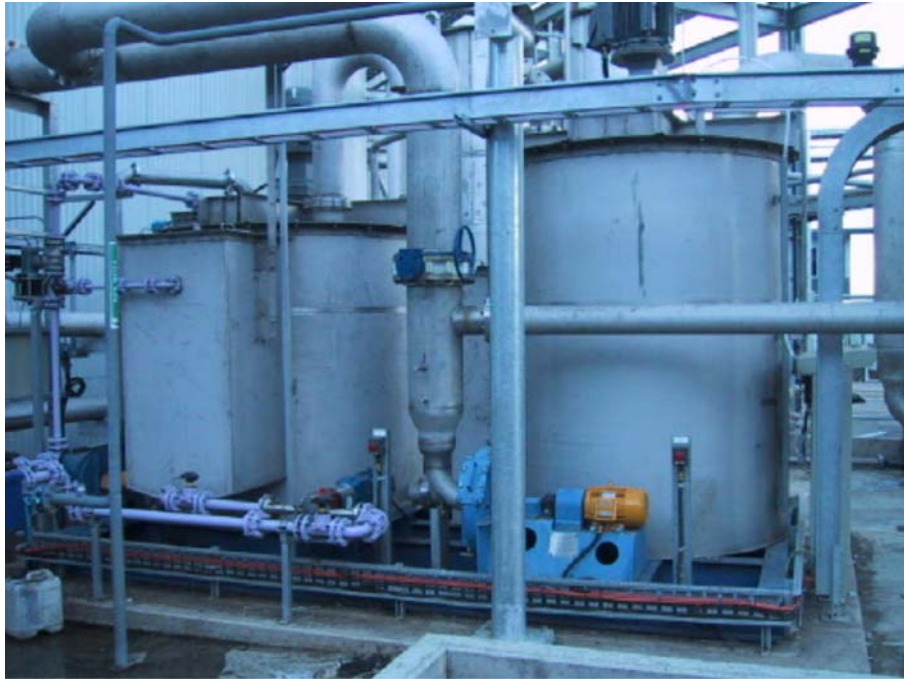
Figure 3: Biogas Purification System at Eastern Creek Processing Plant, Sydney Australia
