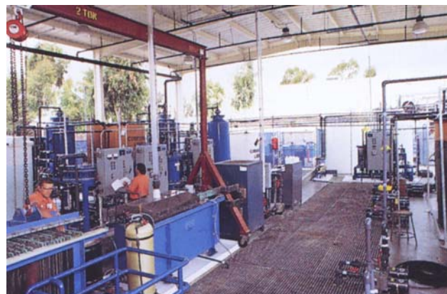
Figure 3 – Copper removal overall system layout
