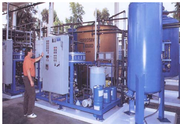
Figure 2 – Copper removal Ion exchange unit.
