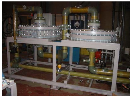
Figure 8: 200gpm SAC: WAC Short Bed Softener
