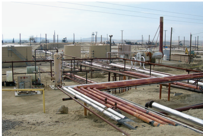
Fig. 1. A complex network of pipes carries steam to and water from Seneca Resources' heavy oil operations in Lost Hills, California.
