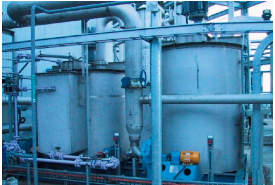
Commissioned in 2005, the GRD Minproc BioGas Purification System handles H 2 S levels ranging from 4000 - 5000 ppmv.
