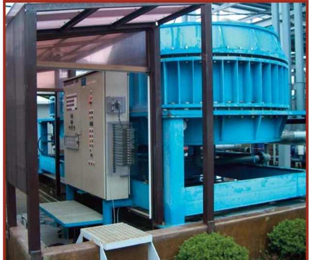
Decationization and Purification Unit (DPU) installed on Capacitor Foil Process in Japan
