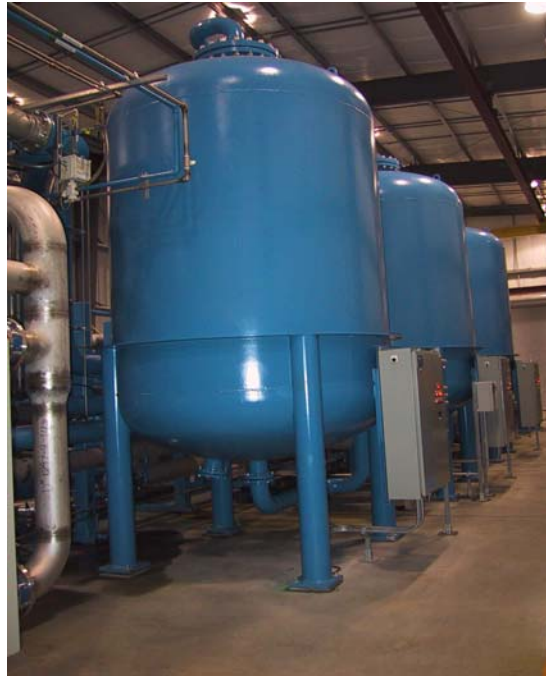
Figure 7: Spectrum Micro-Media Filters at Ontario Power Generation, Pickering Nuclear
